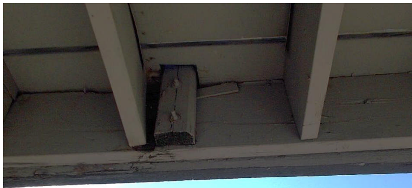
2. Decay at rim joist.
