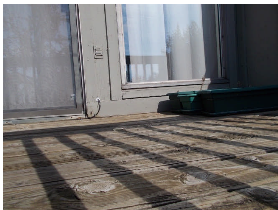
9. 2x6 decking appears weathered.
