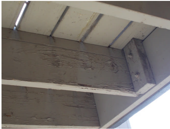
23. Peeling paint on joists.
