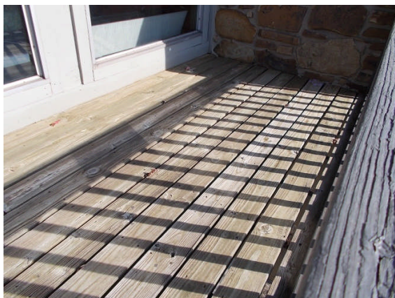
3. 2x6 treated decking; no stain.
