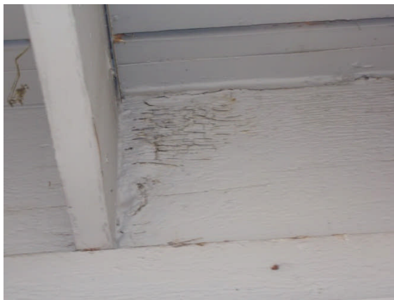
21. Decayed blocking above garage door.
