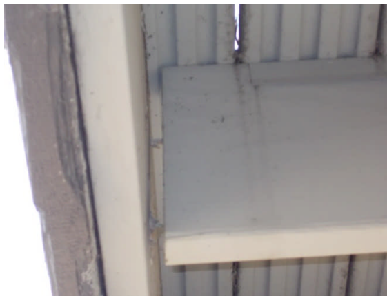
14. Rim pulling away from end of joist.
