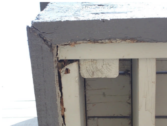
17. Decayed joist at east end.
